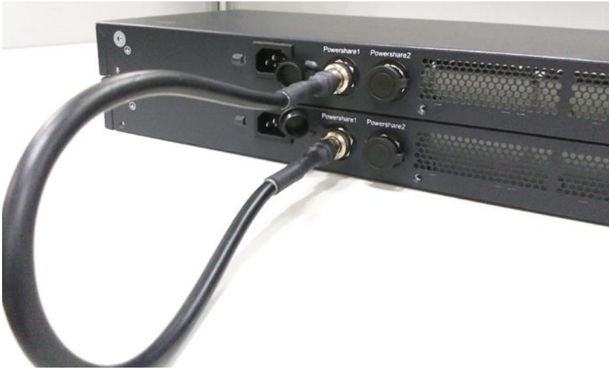
Figure 3-9 Connecting Cables between Two Switches
